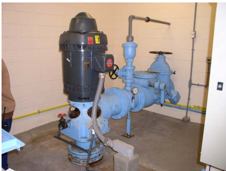
Figure 3.2 Mission Trace Groundwater Well Pump
