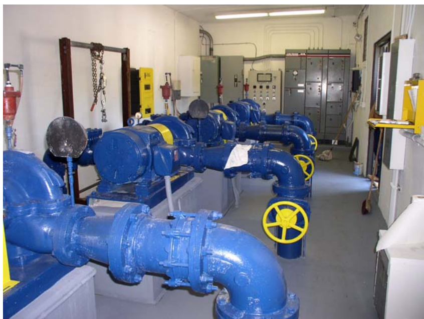
Figure 3.3 Old Jefferson Distribution Pumps
