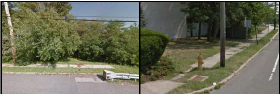
Figure 38: Sidewalks provided are often too narrow, overgrown, and end at poor locations without crosswalks (left: Hooper Avenue/Seaview Village); or have utilities in the right-of-way (right: Hooper Avenue, Bay Harbor) (Google Streetview)
