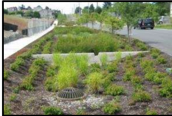
Figure 204: Example of a streetside bioswale ( www.kwalliance.org )
