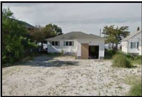
Figure 75: Damaged/Gutted home, Post-Sandy (Google Streetview)
