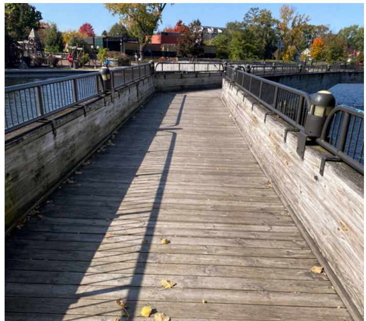
Bridges spanning the width of the pond make for great viewing experiences of the water and surrounding scenery.
