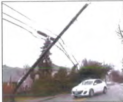
Electrical Service Interruption
