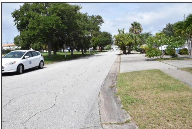
Cracked Pavement near intersection of Jefferson Ave. and Poinsetta Ave.
