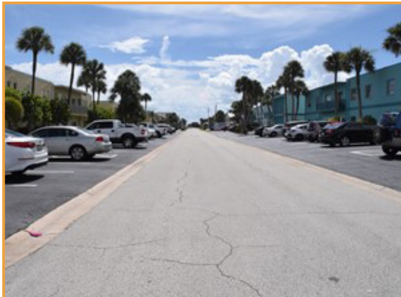
Cracked pavement and parking areas against roadway on Taylor Ave
