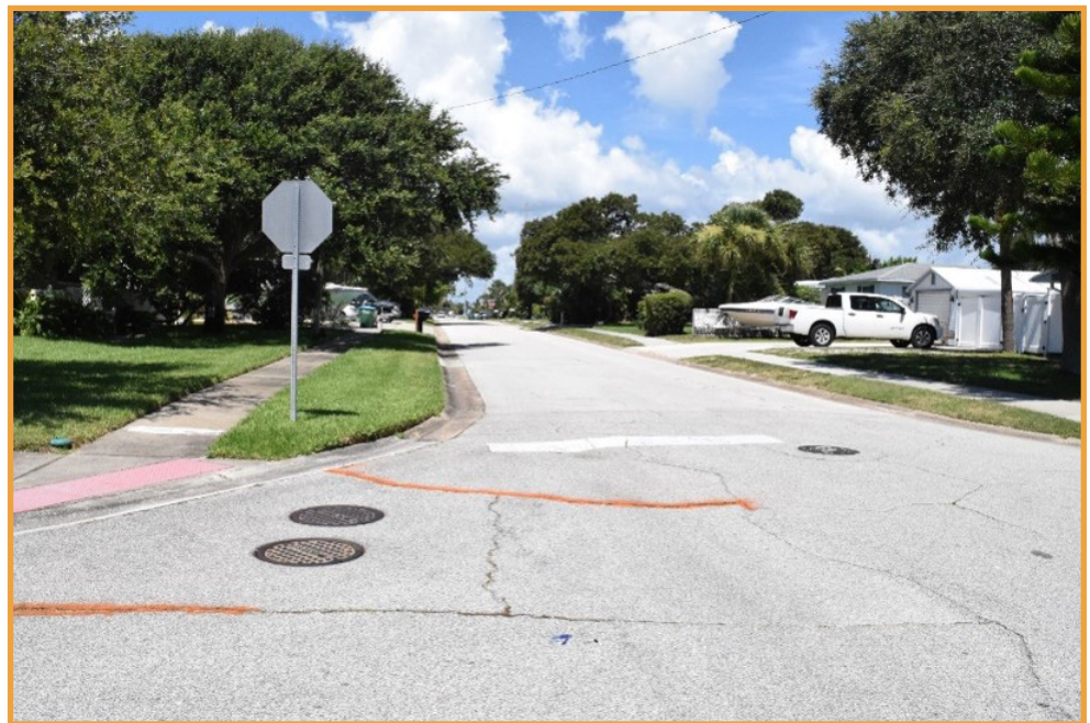
Photo of pavement cracking at the intersection of Orange Ave and Buchanan Ave
