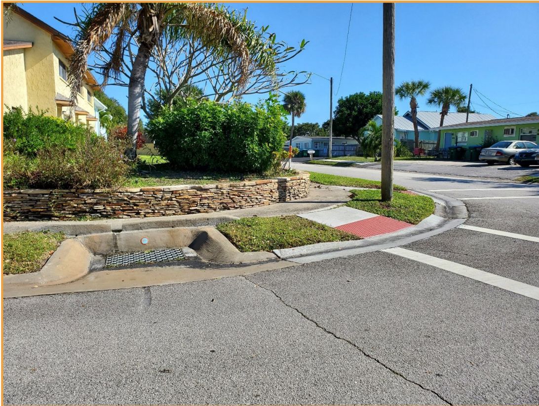
Photo of curb inlet and ADA accessible crosswalk at Poinsetta Ave and Pierce Ave
