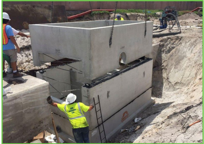
Figure 16. An example of a second-generation baffle box. Credit: St. Johns River Water Management District.
