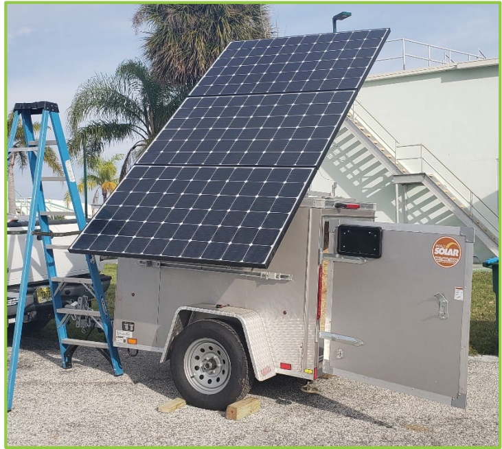
Figure 23. Mobile Solar generator (2019).
