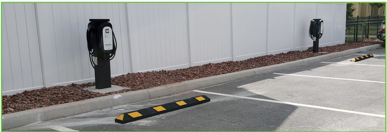
Figure 29. Electric vehicle (EV) charging stations.
