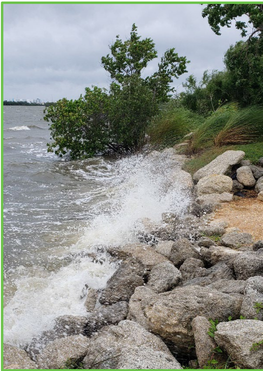
Figure 6. Wave action off the lagoon at Banana River Park's coquina seawall during 2019's Hurricane Dorian.
