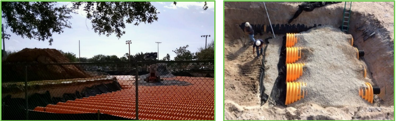
Figure 18. Exfiltration projects, Canaveral City Park (left) and City Hall (right).
