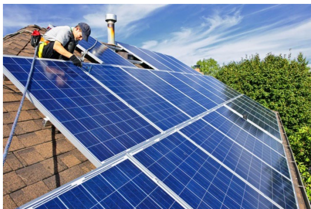
Figure 1. Example of a residential rooftop solar array.
