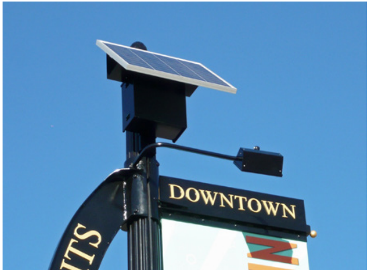
Smart infrastructure efficiently lights wayfinding signage
