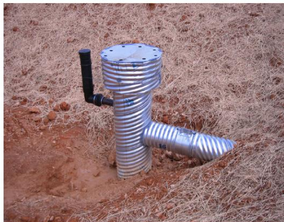
Figure 7.31-6 Dewatering device on Riser with Trash Rack
