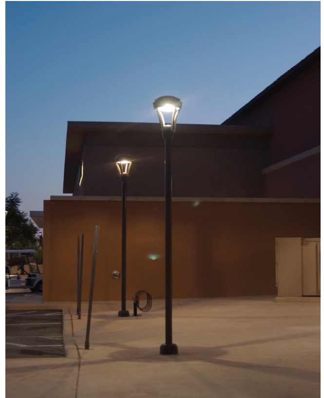
This shielded outdoor lighting fixture provides visibility where it is needed without unwanted light pollution
