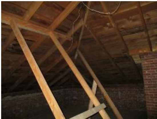
Picture 5: Roof truss pocketed into brick wall
