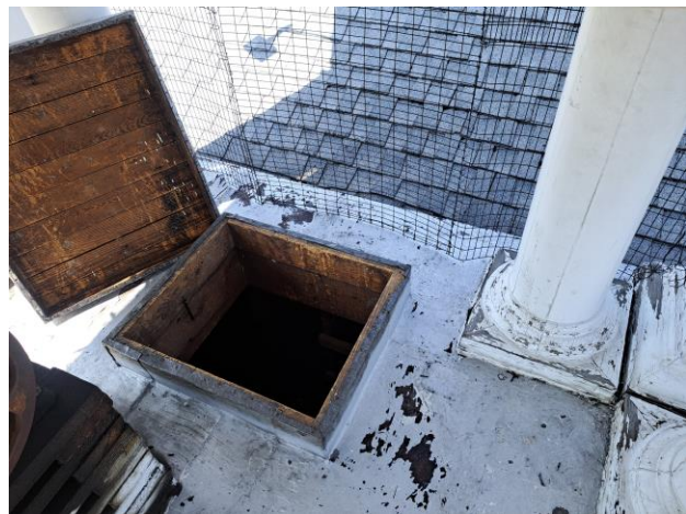
Failed exterior paint finishes at the bell tower. (A&E Design)
