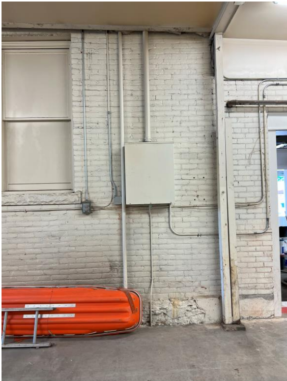
Figure 3 – CT enclosure in North Apparatus Bay
