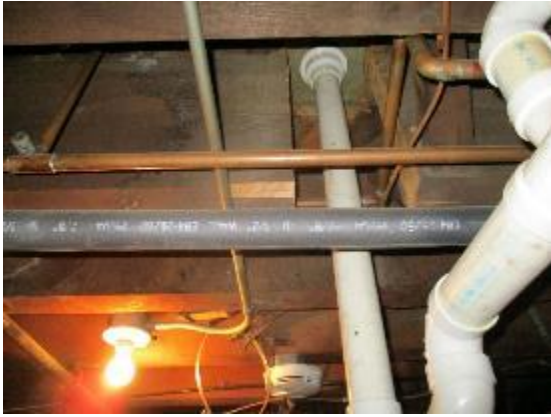
Picture 1: Cut joist, main floor
