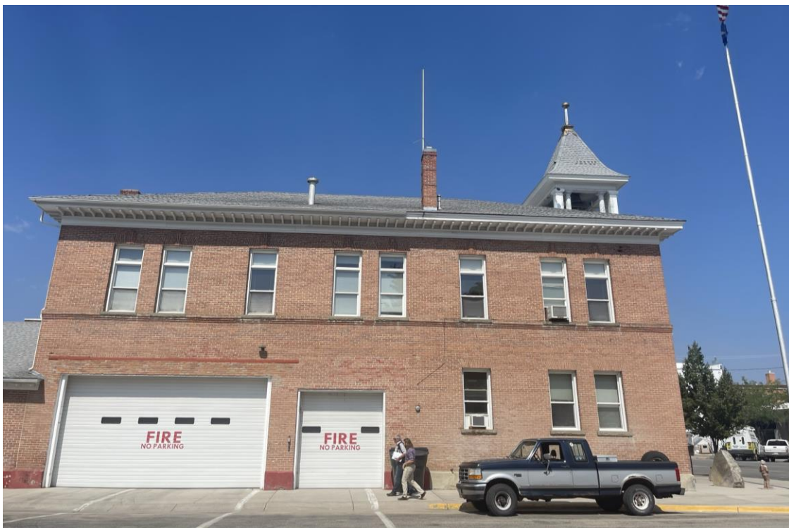
Cladding on historic window frame, non-historic window unit, and deteriorated finish on cornice and fascia. (A&E Design)
