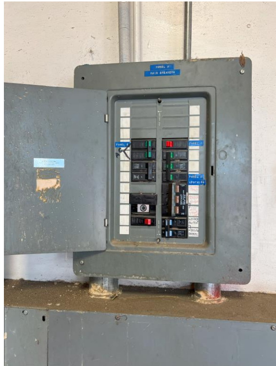
Figure 4 – Main distribution panel A
