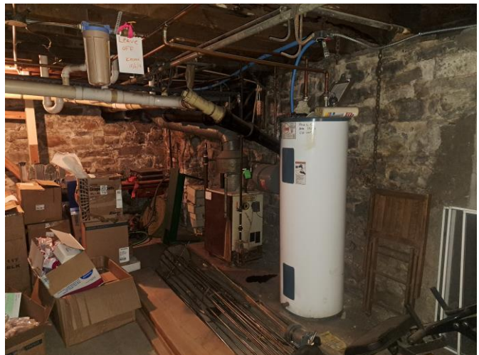
Basement mechanical space. (A&E Design)
