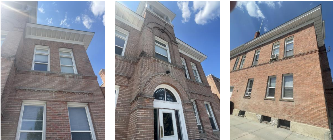
General masonry staining and discoloration. (A&E Design)
