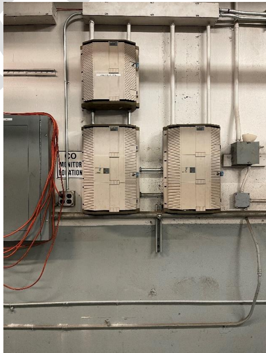
Existing Boiler BAS Controls
