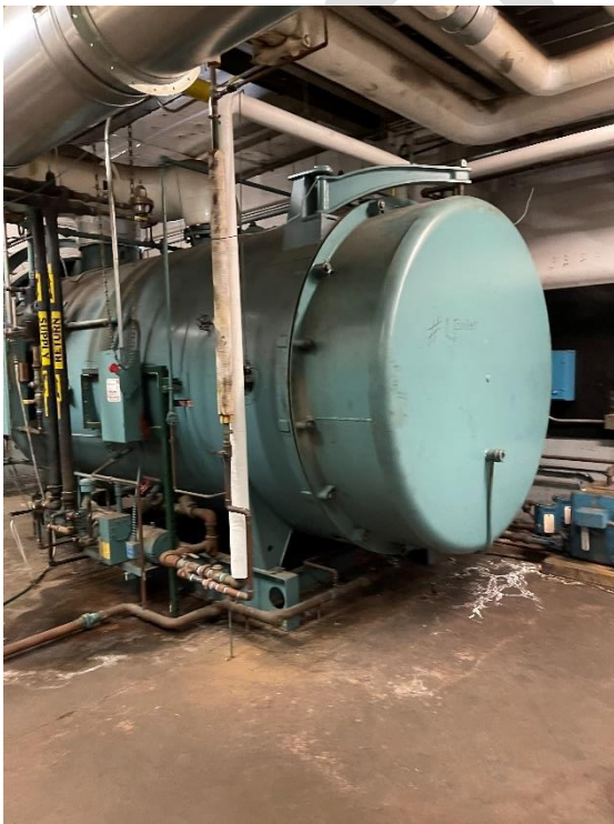
Cleaver Brooks Boiler #3
