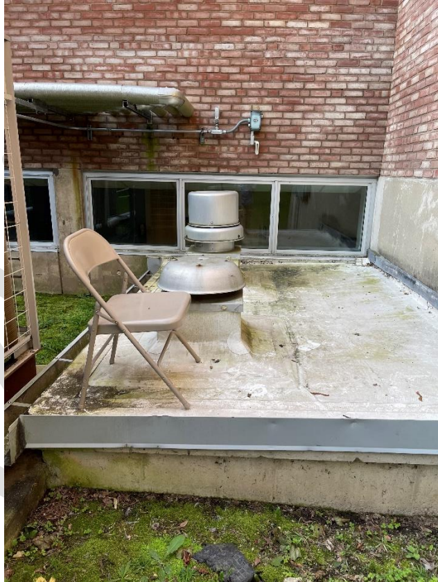
Courtyard (lower level) Exhaust Fans
