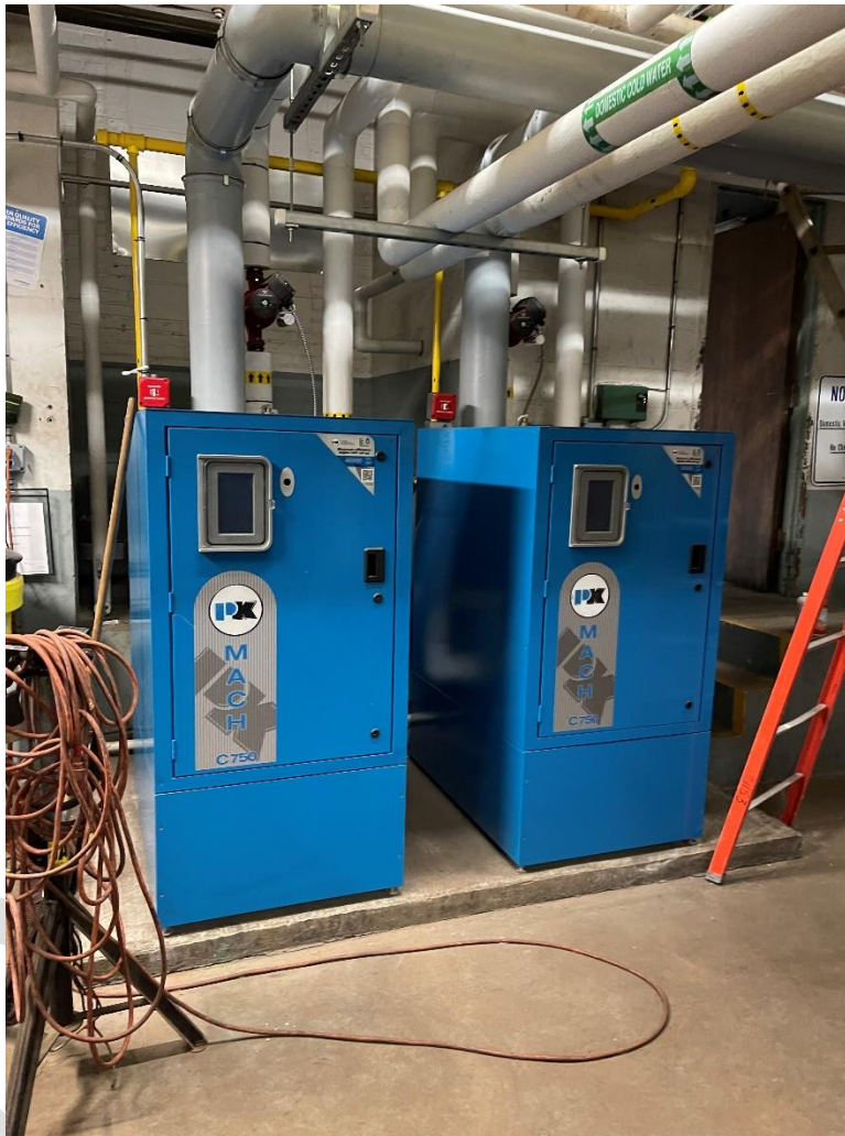
(2) Domestic Hot Water Heaters
