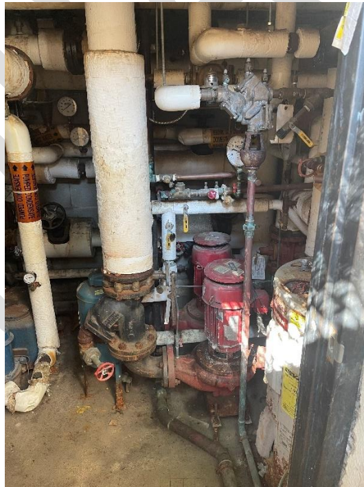
Perimeter Heating Pumps
