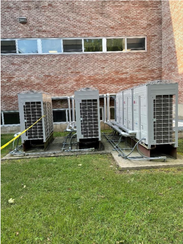
Courtyard Condensing Units
