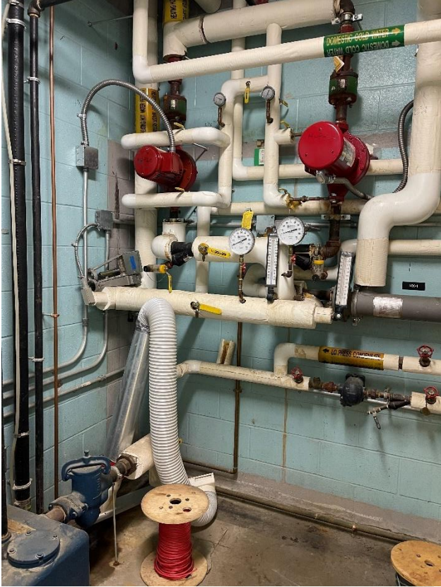
Perimeter Shell & Tube and Pumps (HX-1)
