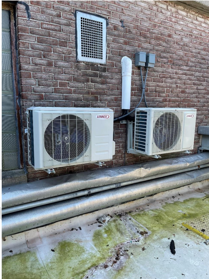
Rooftop Air-Cooled Condensing Units
