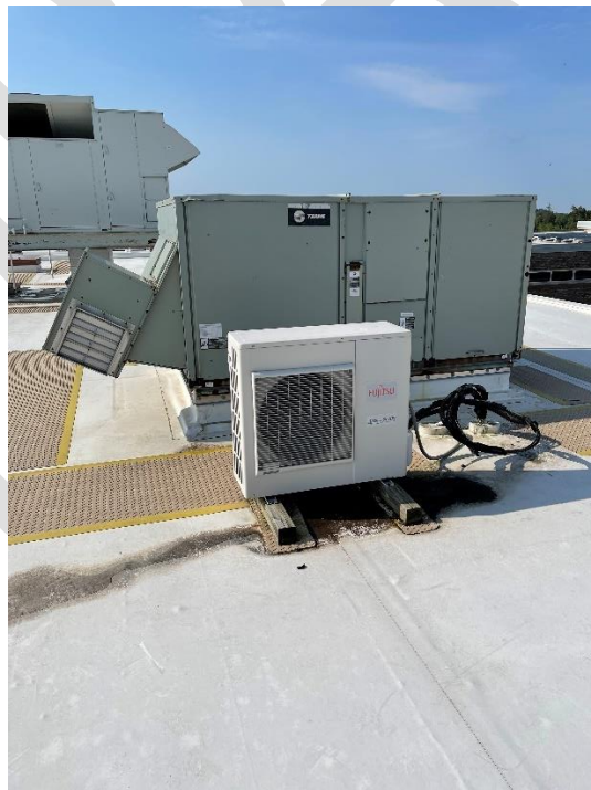
Rooftop Package Unit (Smaller Capacity) & Rooftop Condensing Unit
