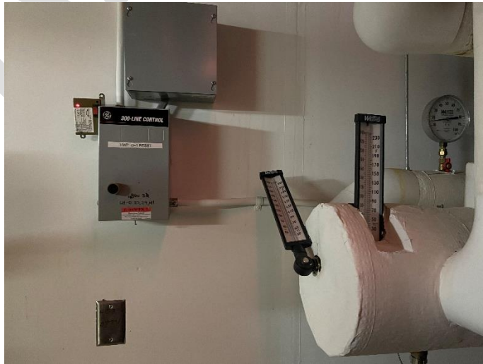
Perimeter Shell & Tube (No Tag)
