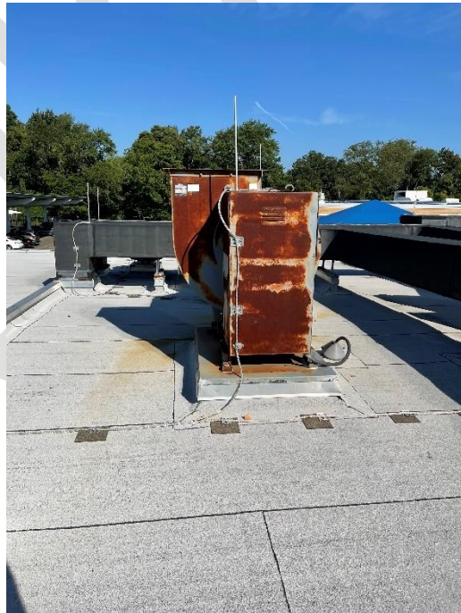
Miscellaneous Exhaust Fans
