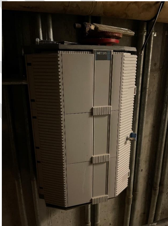
Johnson Metasys Control Panel
