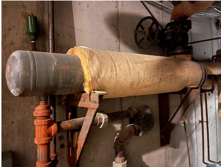
Perimeter Shell & Tube (No Tag)
