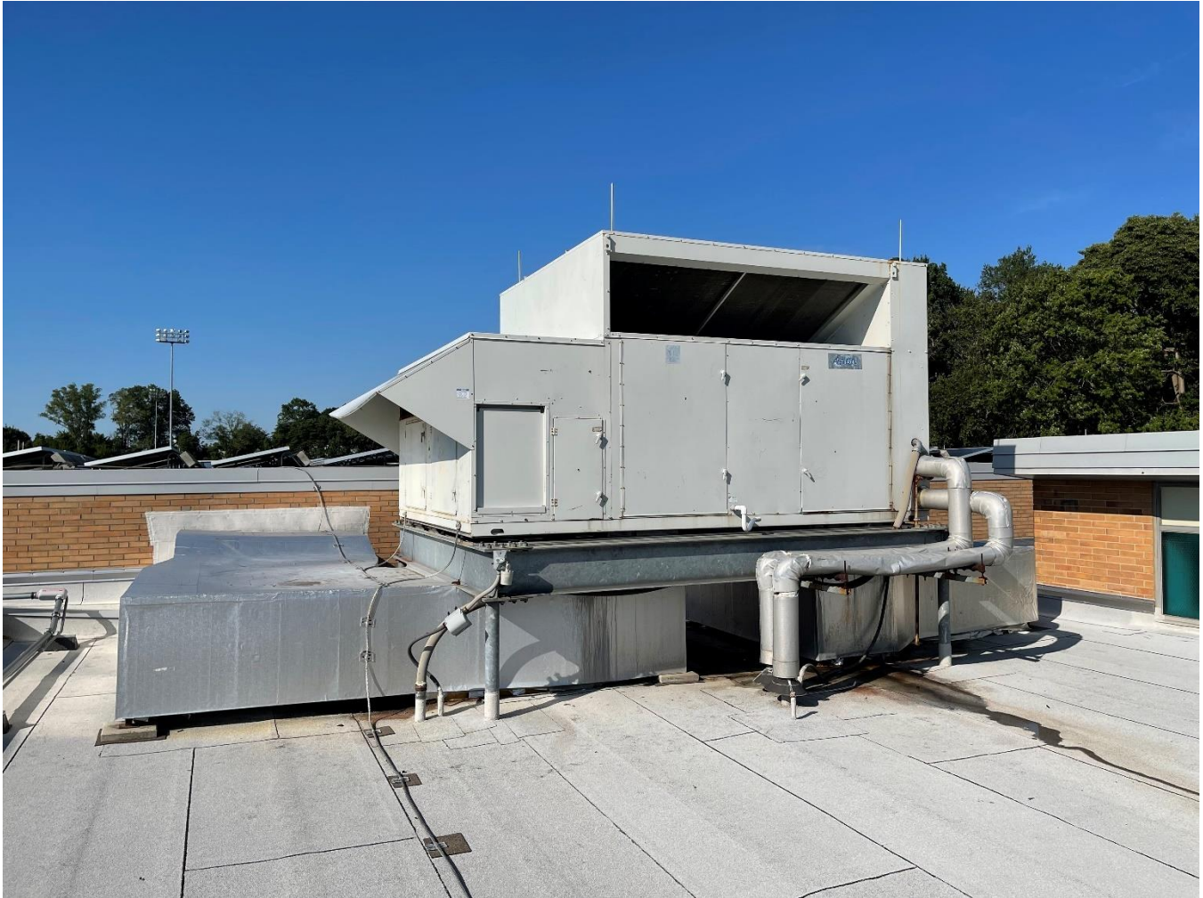
Rooftop Packaged Air-cooled Hot-Water Heat Unit
