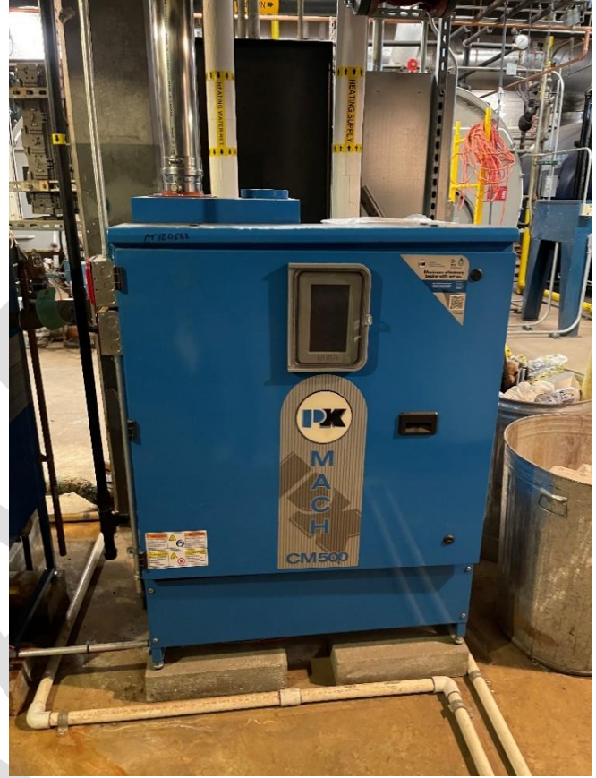
Domestic Hot Water Heater
