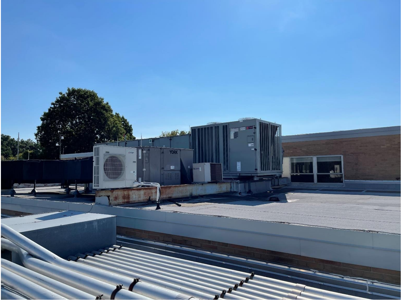
Rooftop Air-Cooled Condensing Unit and Packaged Rooftop Unit
