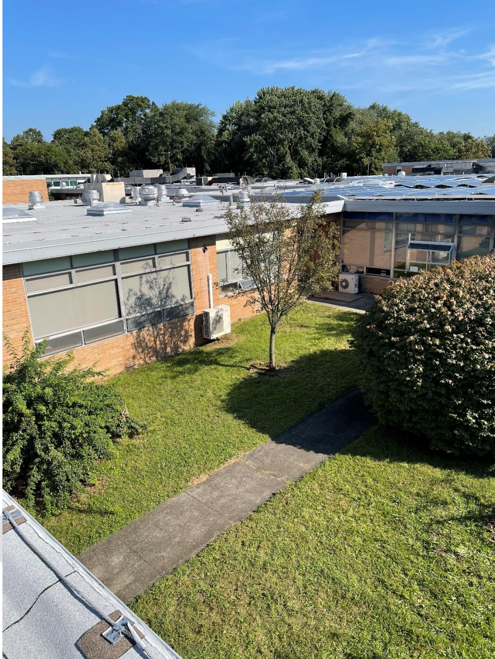
Courtyard Air-Cooled Condensing Units
