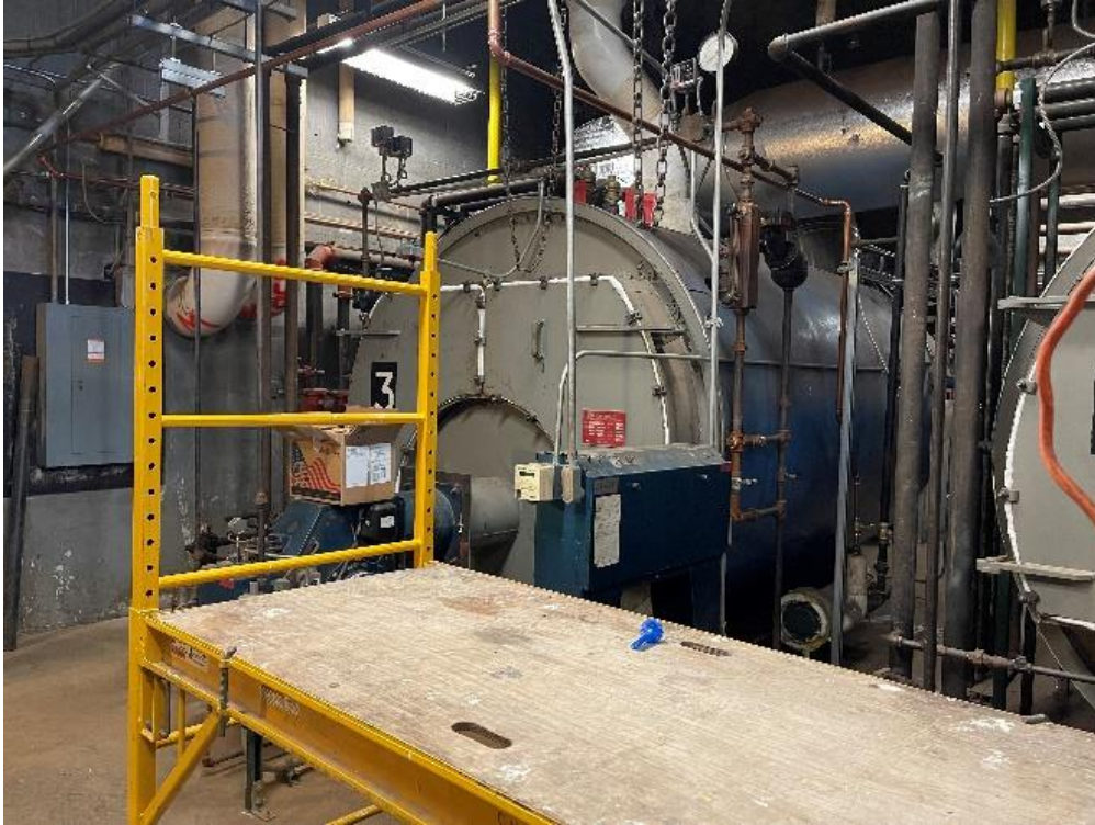
Easco Brooks Boiler #3
