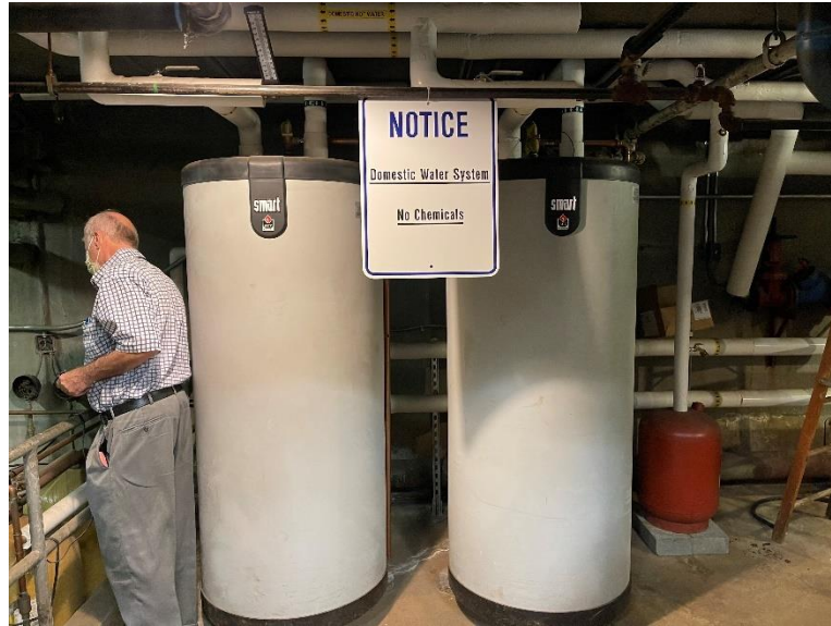
Domestic Hot Water Storage Tanks
