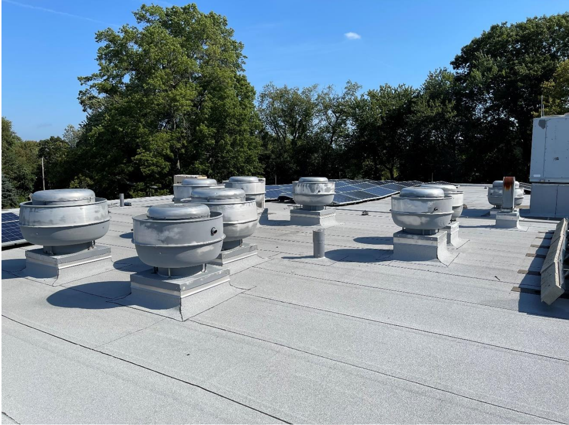
Miscellaneous Exhaust Fans
