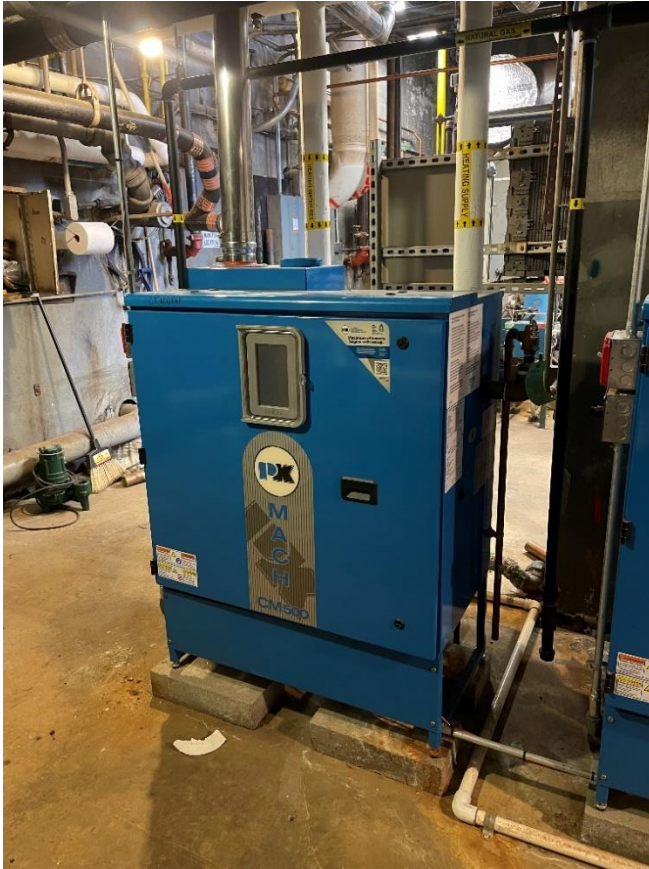
Domestic Hot Water Heater
