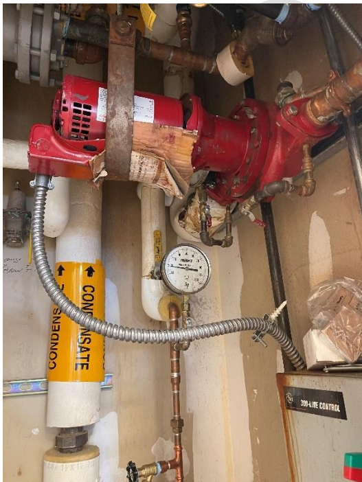
Perimeter Heating Pumps
