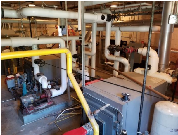
Existing Boilers in Boiler Room
