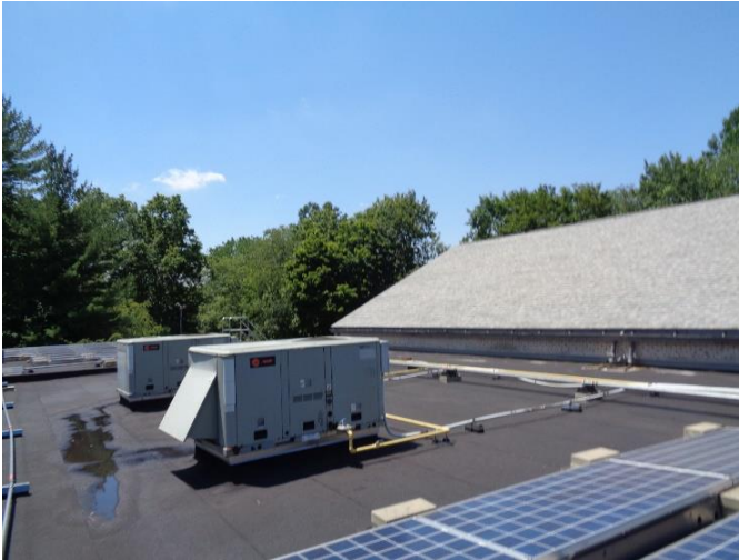
Existing RTU's 4 and 5 to be replaced in 2021
