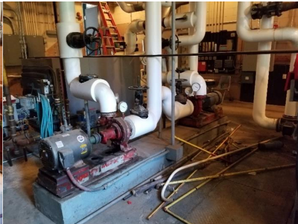
Existing Hot Water Pumps
