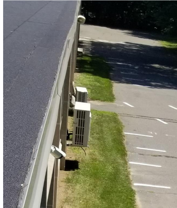
Existing Wall Mounted Mini Split Condenser
