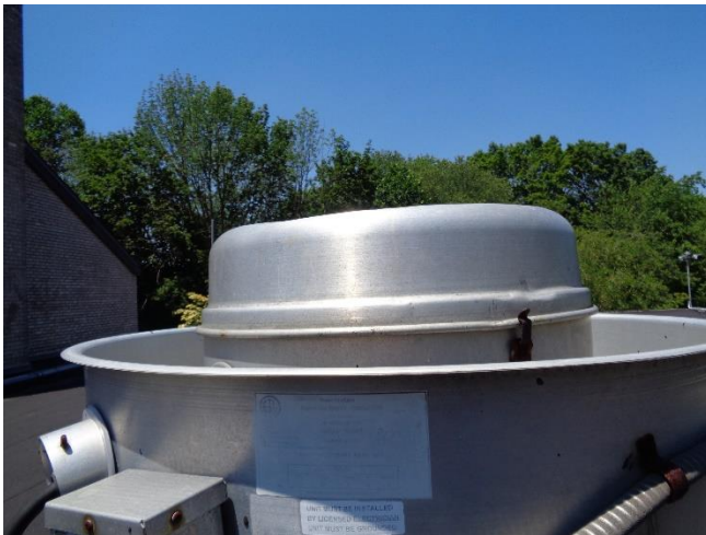
Existing Rooftop Exhaust Fan.
