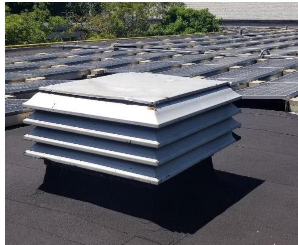
Existing Rooftop Equipment
