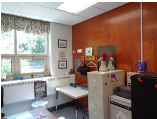
Existing Perimeter Heat
