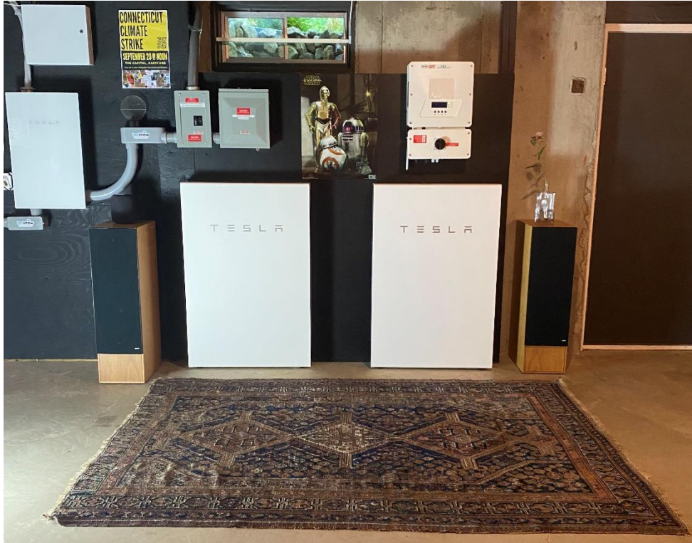
Tesla Powerwall residential backup batteries
