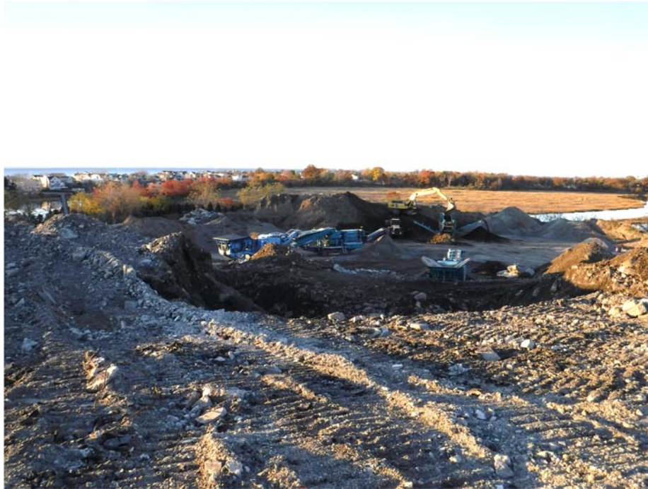
Long-stick excavator in background atop smaller pile of previously screened material. Julian is running material from this pile through one screener and has moved the larger screening operation further to the southeast away from the base of the main pile.
