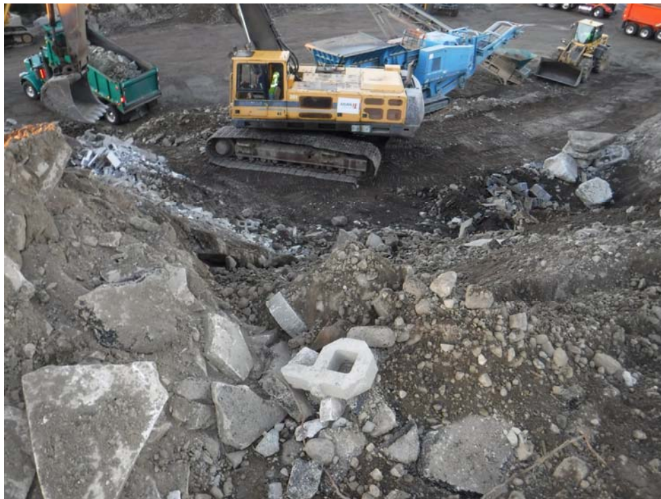
Main pile area taken from atop the pile looking down and facing south.
