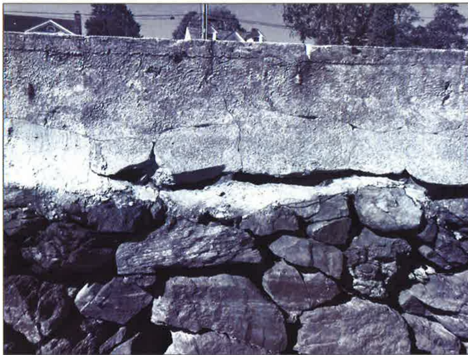
Photograph 11 - Deterioated concrete cap
