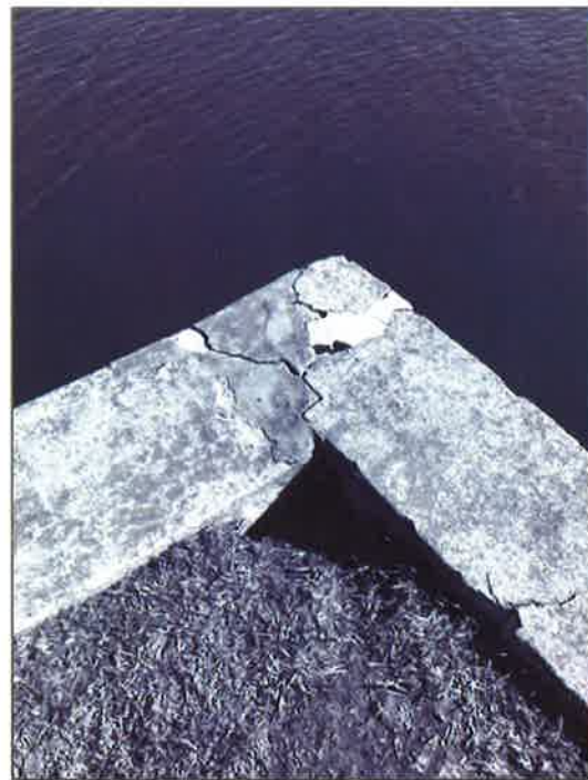
Photograph 5 - Cracking and sinkhole at corner STA 0+96
