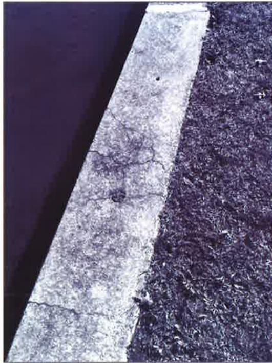
Photograph 4 - Typical cracking in concrete cap
