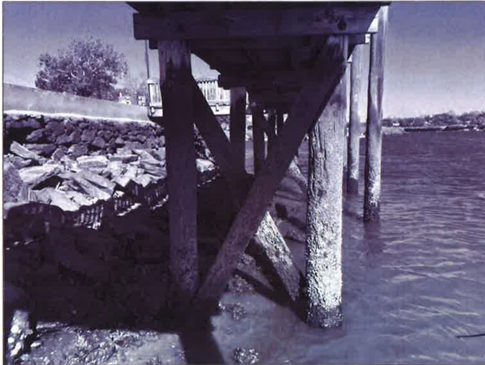
Photograph 24 - Typical damage of the cross bracing
