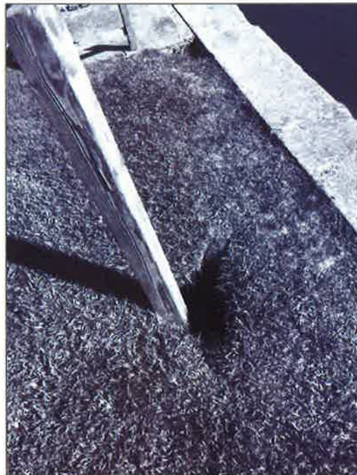
Photograph 7 – Sinkhole at STA 1+02 and shown rotation of concrete pad for bench.
