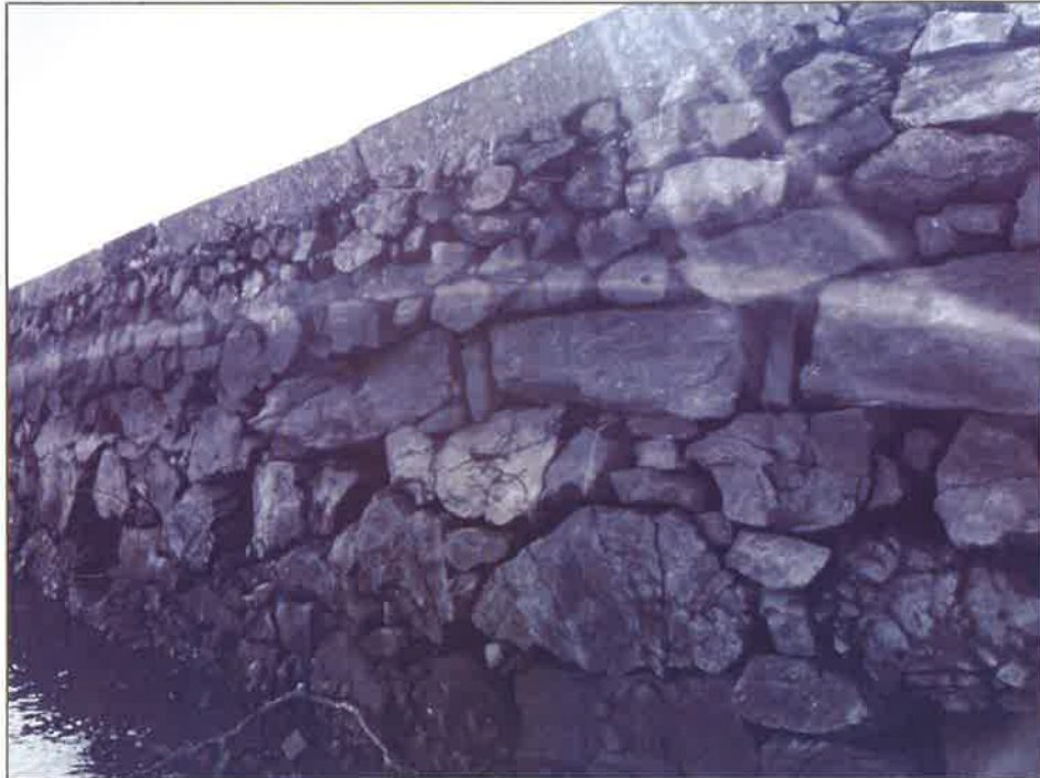
Photograph 6 – Areas of missing stone and outfall location circled in red
