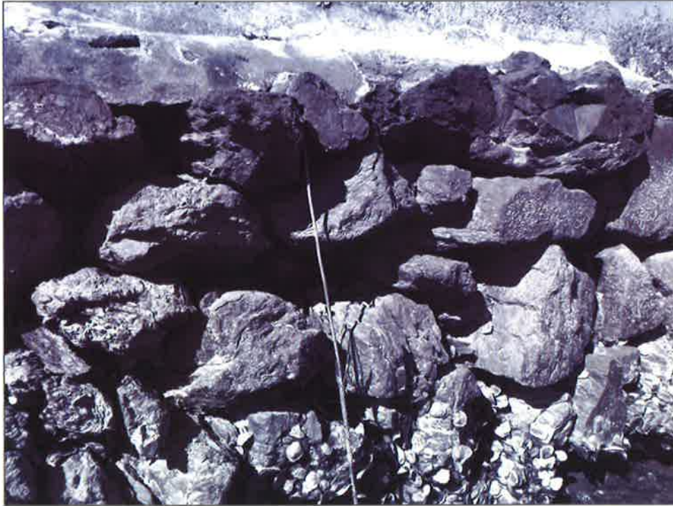
Photograph 18 – Seawall voids at STA 2+27
