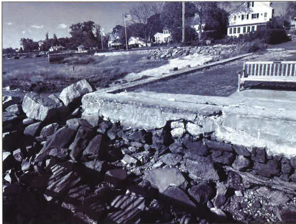
Photograph 19 – Poor condition of the concrete cap and dislodged stones STA 2+73-2+95
