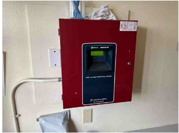
Fire Alarm System
