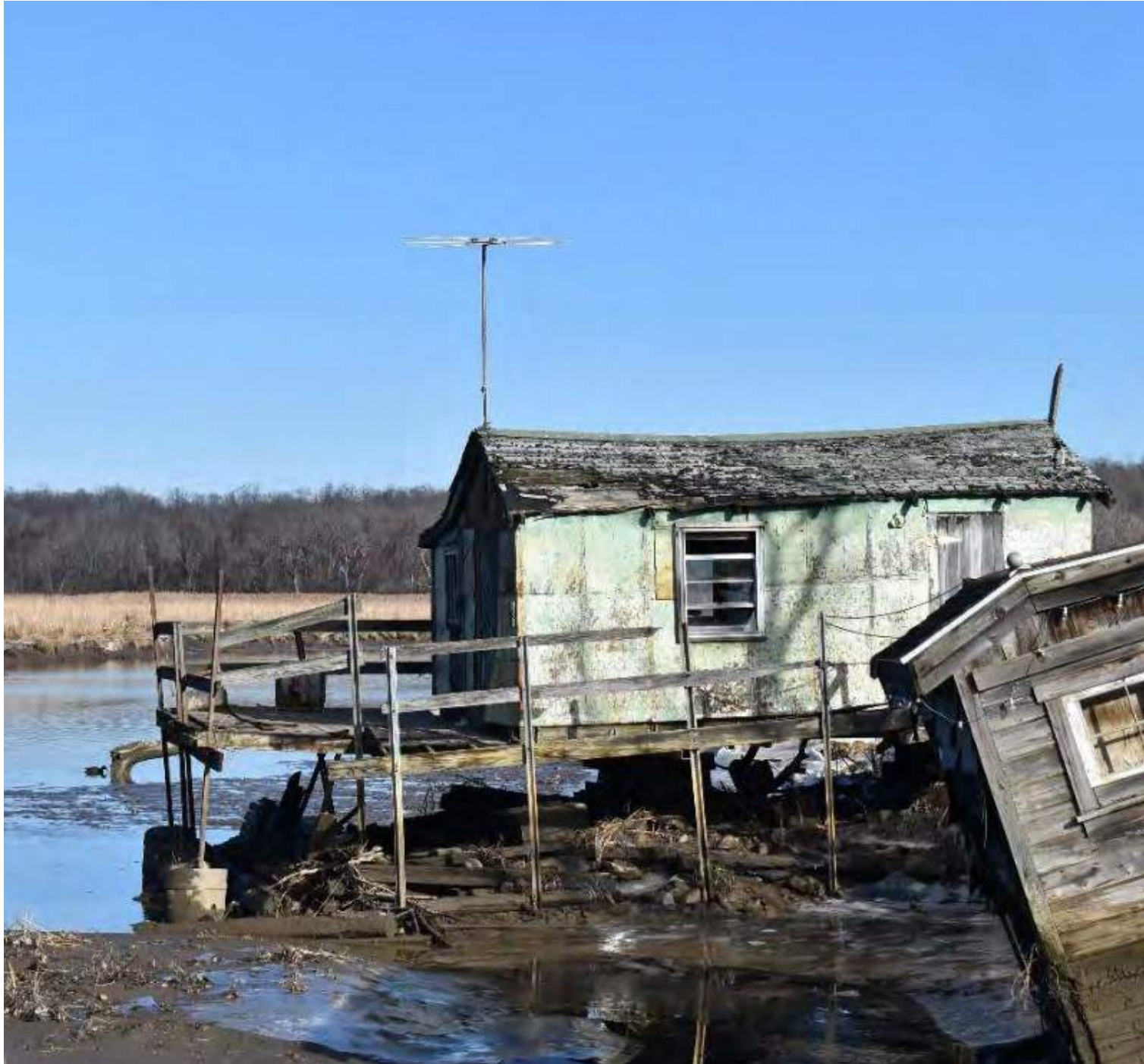
A. SHPO recommends Building 8 be mothballed. However access for any kind of remediation is a challenge.
