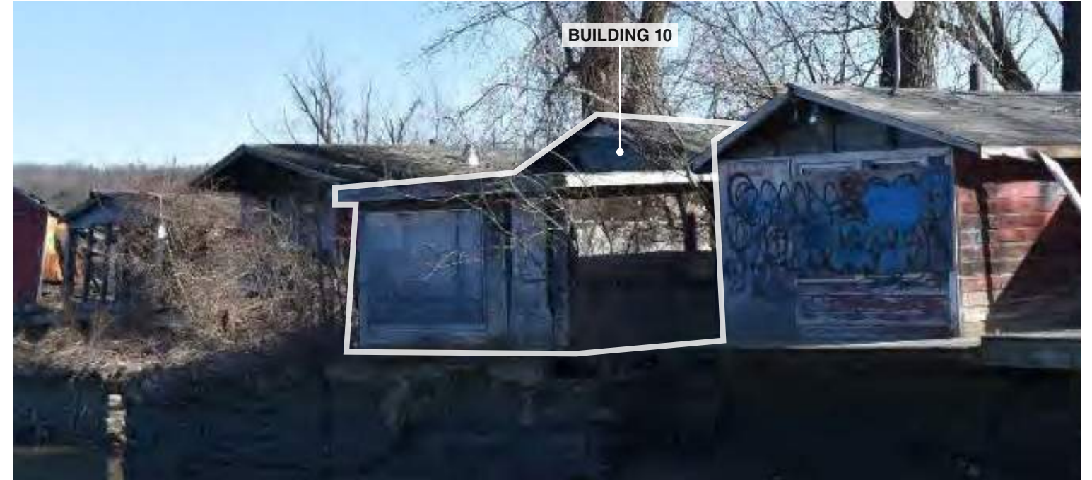
B. Building 10 to be further studied as a candidate for rehabilitation. Image source: Hudson Cultural Services, January 2024.
