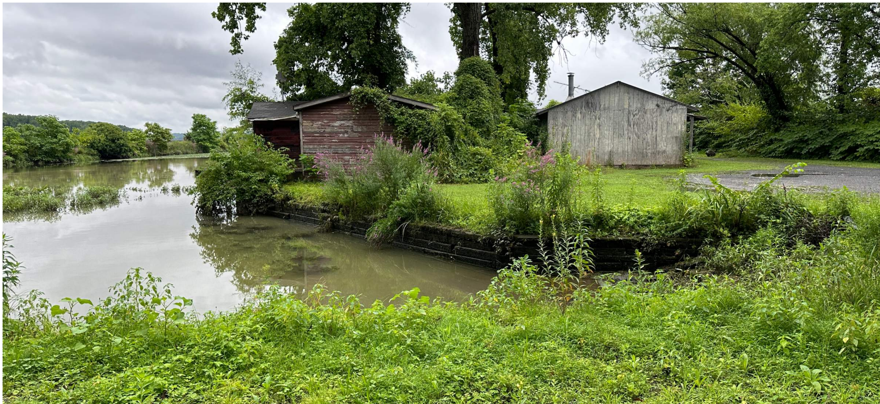
The existing boat launch with a timber bulkhead in decline. The depth and pitch of the ramp are reported to be too shallow for easy water access.
