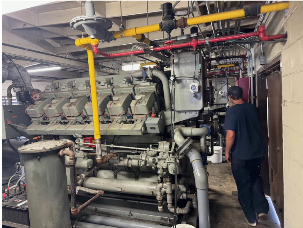
Hamilton Pump Station (2024)
