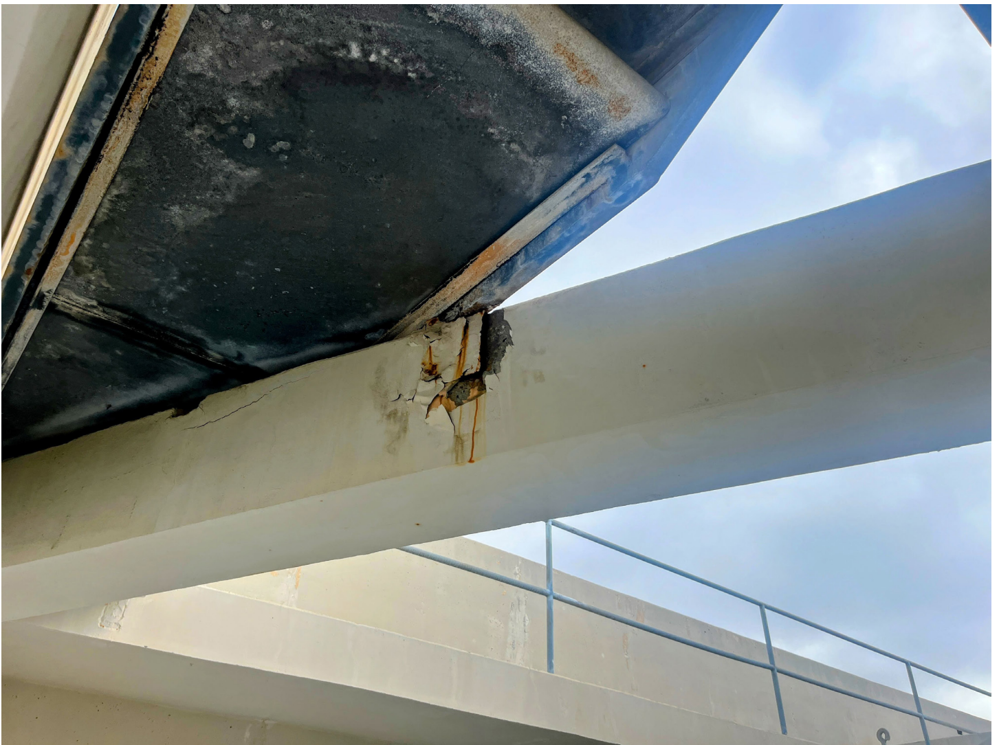
Wear and tear presents structural issues at a City facility
