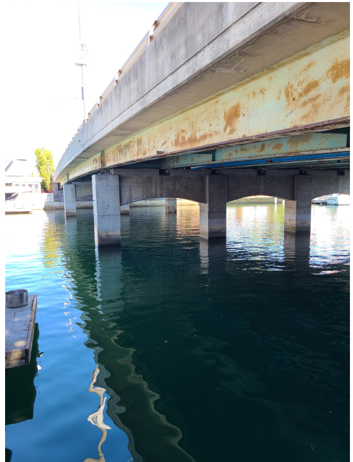
Girders Rust at Admiralty Drive Bridge (2023)
