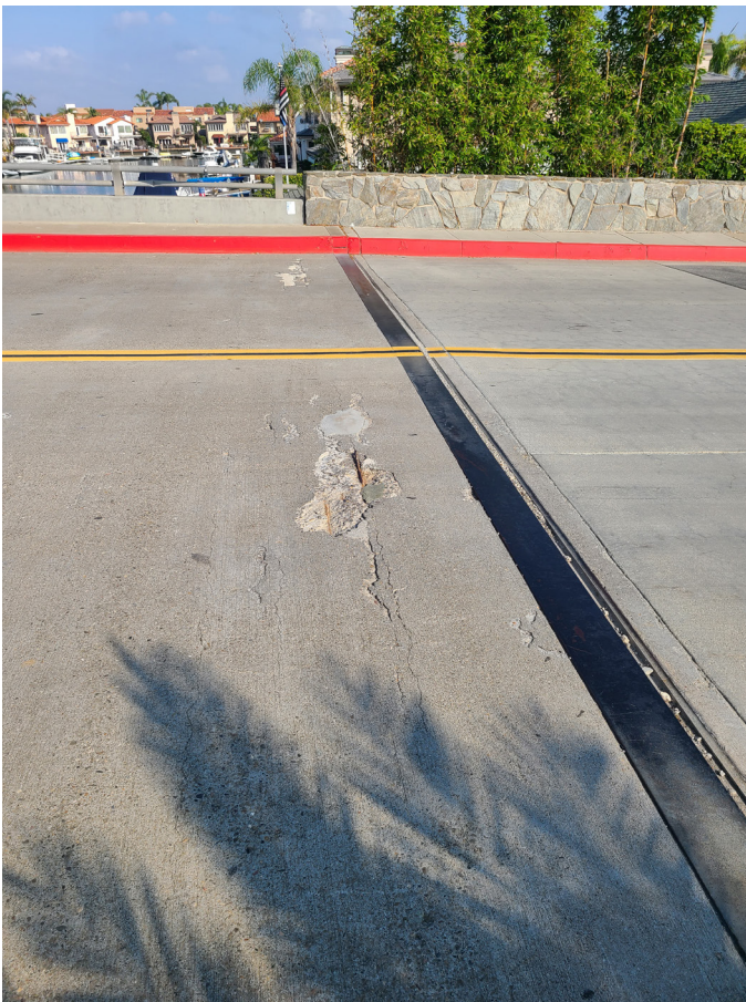
Deck Cracks at Admiralty Drive Bridge (2023)
