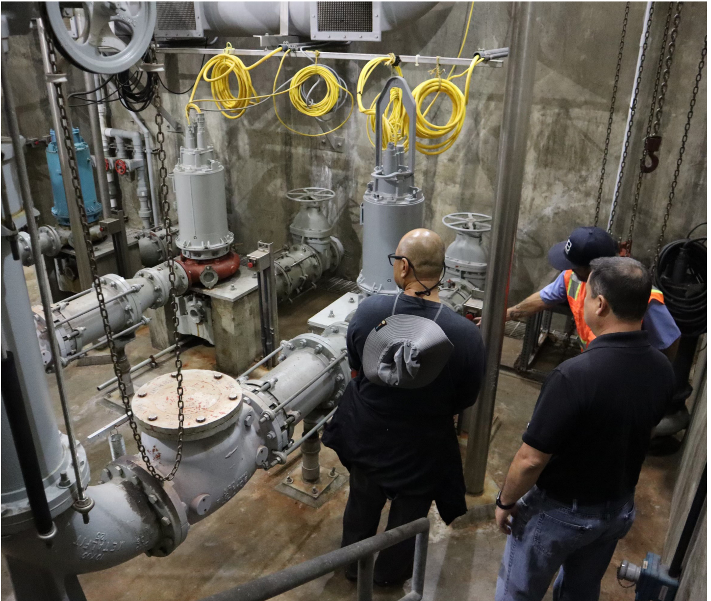
An infrastructure tour inspects D Station, the City's largest wastewater lift station
