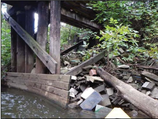
Photo 18: Large debris under railroad trestle
