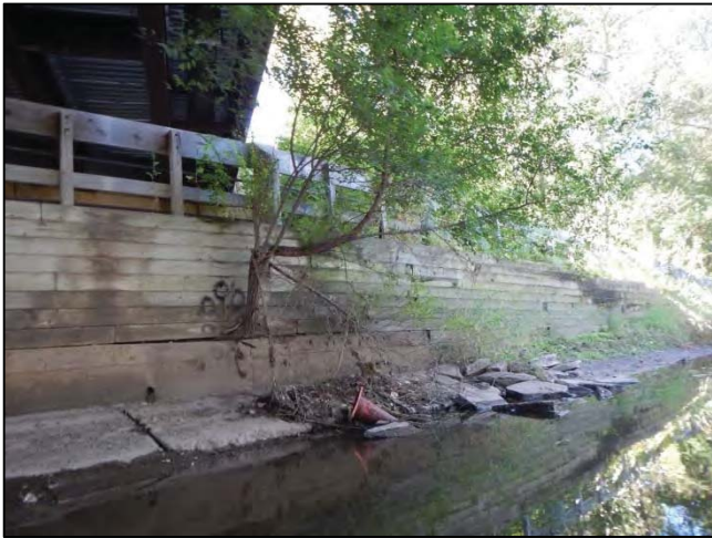
Photo 2: Tree growing under the wall of the Lansing River Trail
