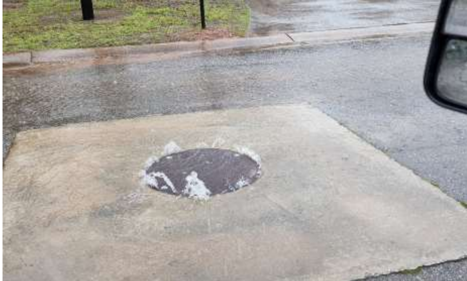
Sanitary sewer overflow in Creekside Subdivision due to I/I
