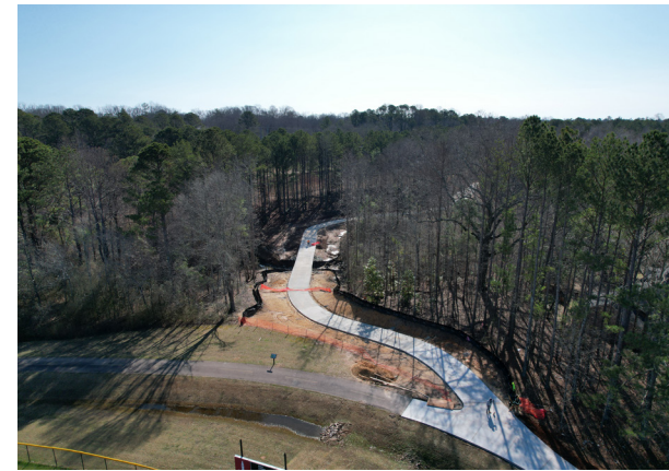
Above: New Construction on the latest segment of The Thread near the George Harris Baseball Fields.
