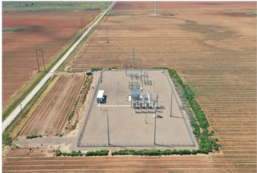
Typical operational Project Substation
