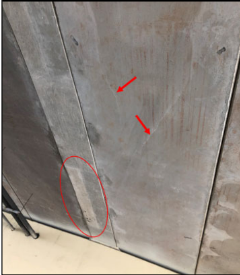
Photo Showing Minor Cracking/ Efflorescence and Previous Repairs at Underside of East
