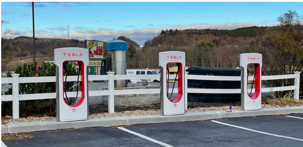
EV charging station in Lawrence Township, Clearfield County
