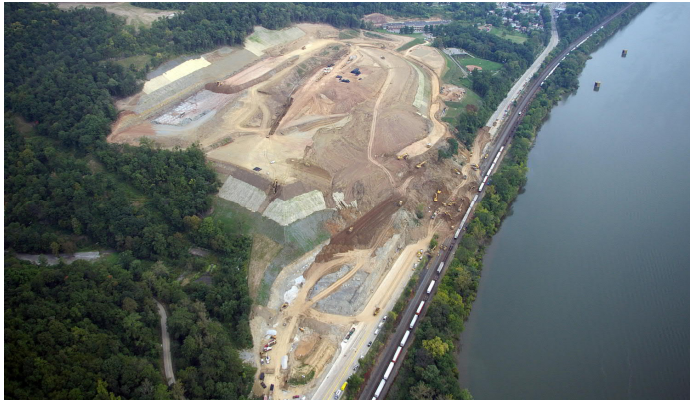
Geosyntec's construction phasing plans were critical to managing interim stability and stormwater control.
