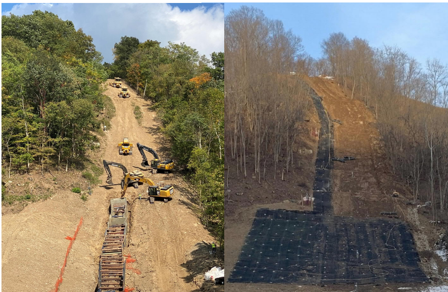
Geosyntec designed and provided onsite engineering support for the stress relief excavation and installation of soil nail and mesh system to mitigate the impact of landslides on a natural gas pipeline
