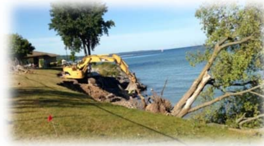
Erosion in Bayfront Park, September 2019
