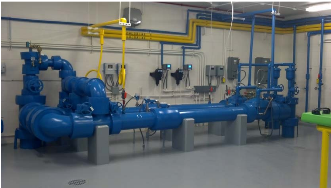
A typical well in the City of Petoskey, where your water is treated and pumped into the water pipes.
