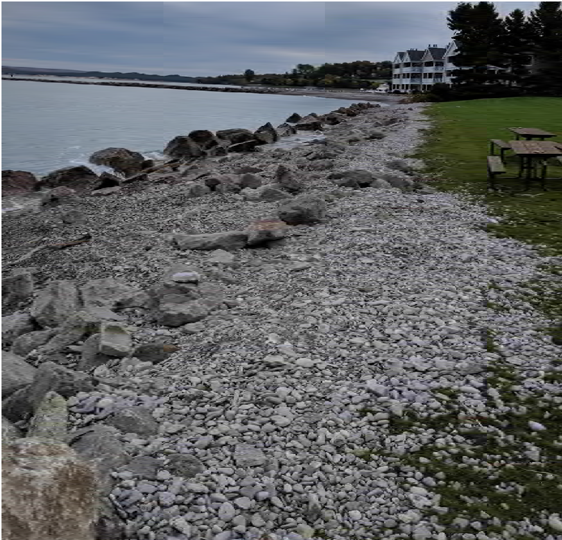
Figure 2.17: Damaged Shoreline Revetment Structure (Baird, 15 October 2019)
