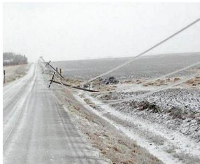
Figure #110 Downed Powerlines
