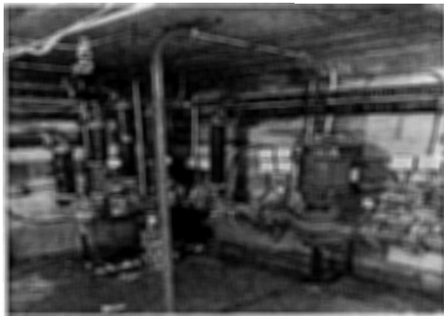
Photo 4: Fire Sprinkler Riser
