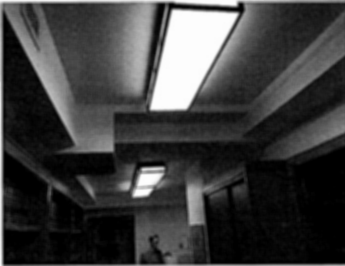
Photo 1: Corridor with Surface Mounted Fluorecent fixtures prior to renovation
