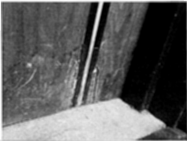
Photo 7: Damage to wood door veneer
