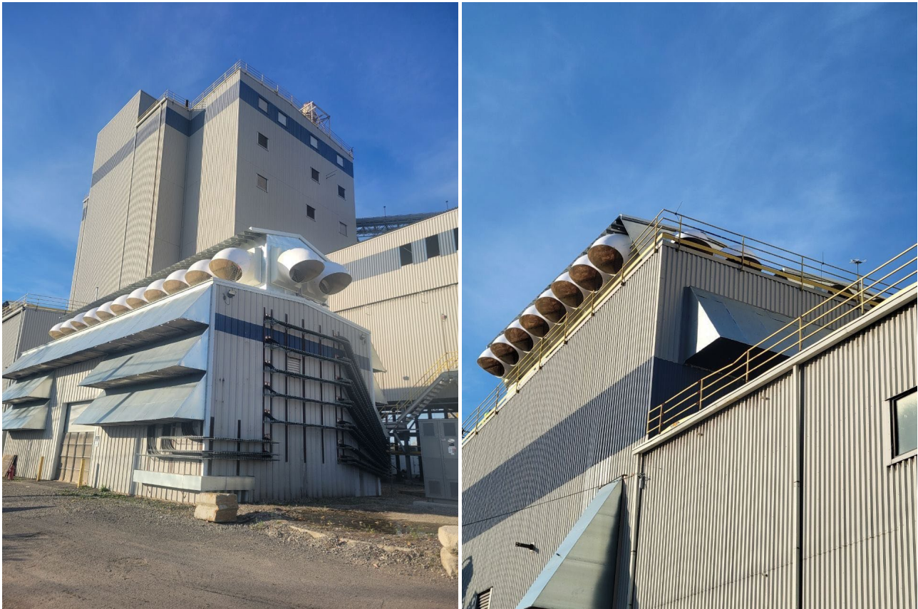
Figure 4 Exhaust Fans Hoods/Cones Installed on POD1 (right) and POD2 (left) Server Buildings
