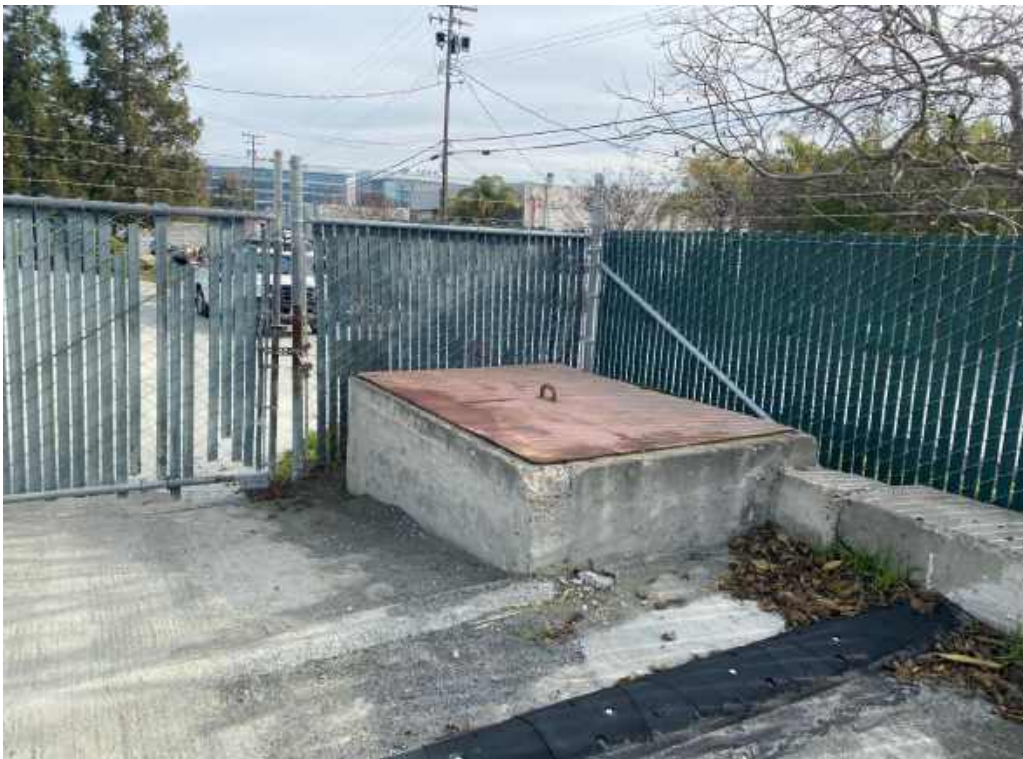
Photo 14: View of storm drain pump, operated by the City of San Carlos, facing east.
