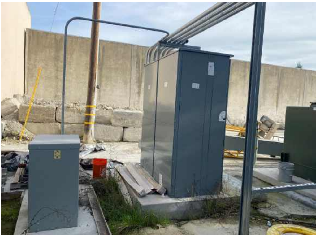
Photo 8: View of the transformers and switch gear, facing southeast.
