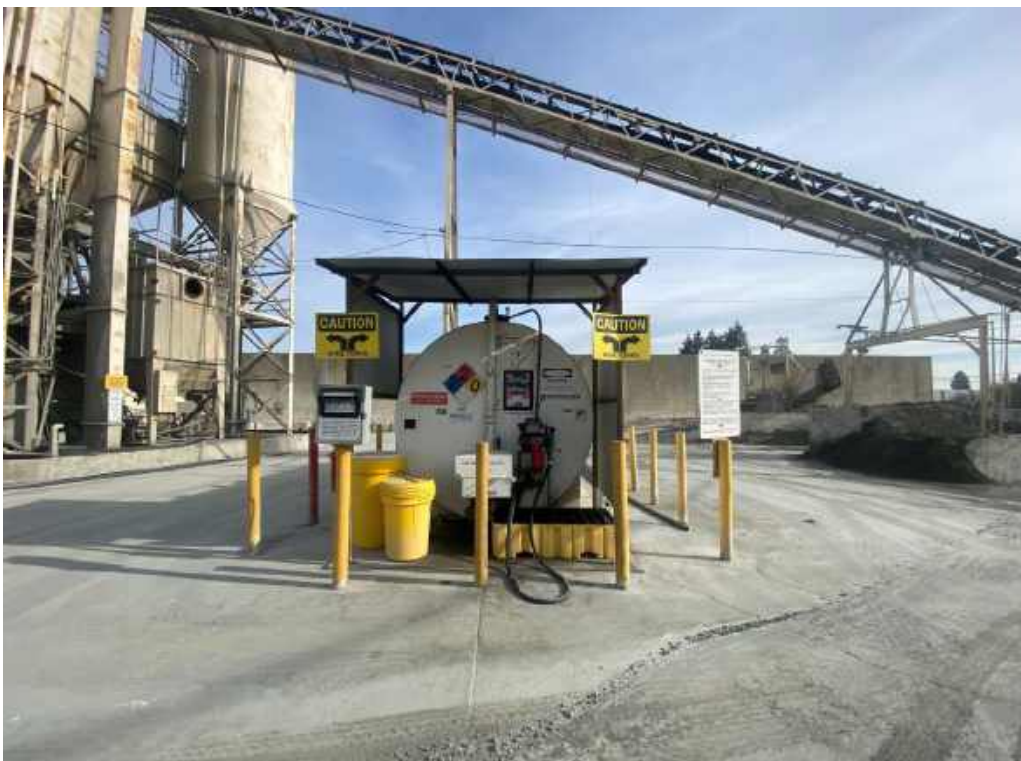
Photo 12: view of the bio-diesel above ground storage tank and batch plant conveyor, facing northeast.
