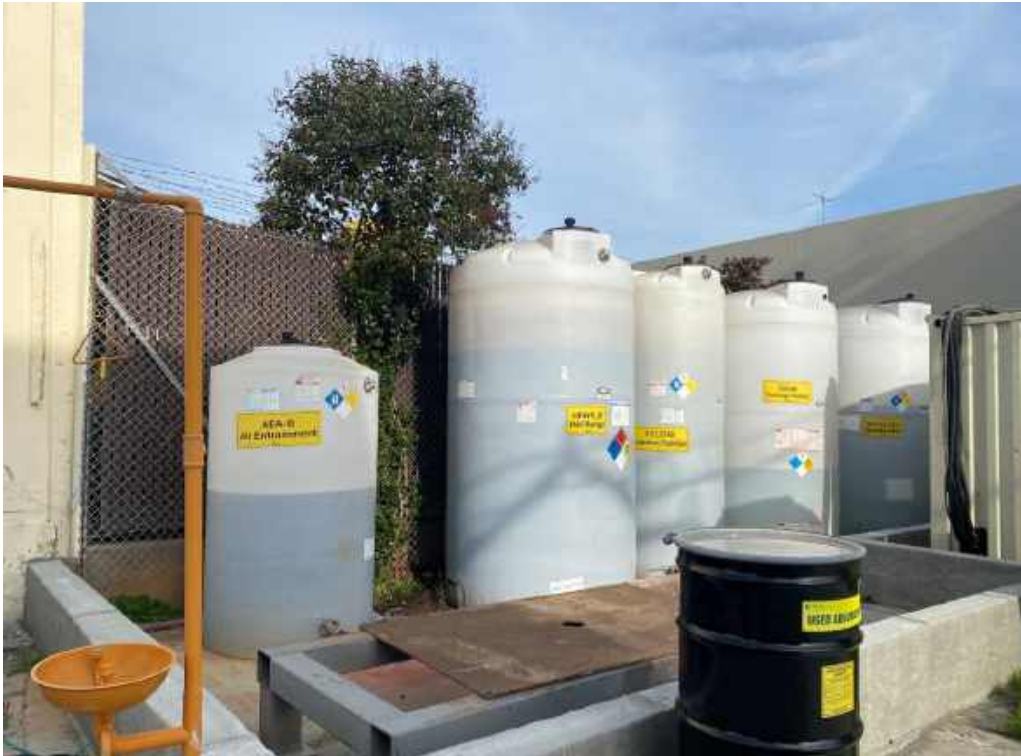
Photo 7: View of the admixture tanks and drum, facing north.
