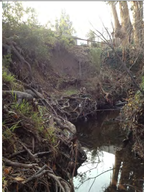
Photo 43. Taken upstream of 6th Avenue adjacent to 1000 O'Neill Avenue, facing upstream The channel is incised. There are signs of bank scour and failure along the right bank (facing downstream) shown on the left in the picture above. The channel is undermining the right bank below existing root ball systems.
