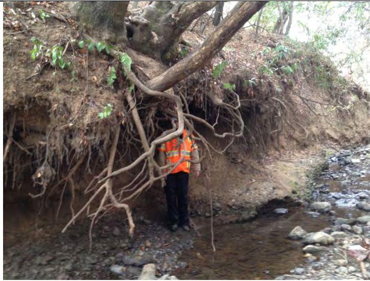
Photo 23. Taken approximately 2,440 ft upstream of the culvert crossing at Chula Vista Drive facing upstream and the right bank The channel has undermined the right bank to a height of approximately 6 ft.
