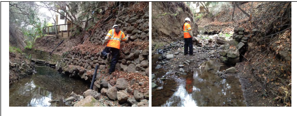
Photo 22. Taken approximately 2,470 ft upstream of the culvert crossing at Chula Vista Drive facing upstream Rock barriers have been placed along the left bank. There are signs of scour at the downstream end of the rocks and channel has undermined the rocks. Upstream of the rocks, sacked concrete and a concrete apron have been placed. The concrete and sacked concrete are also being undermined. The right bank is nearly vertical.
