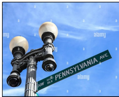
Cameras installed on decorative streetlamp
