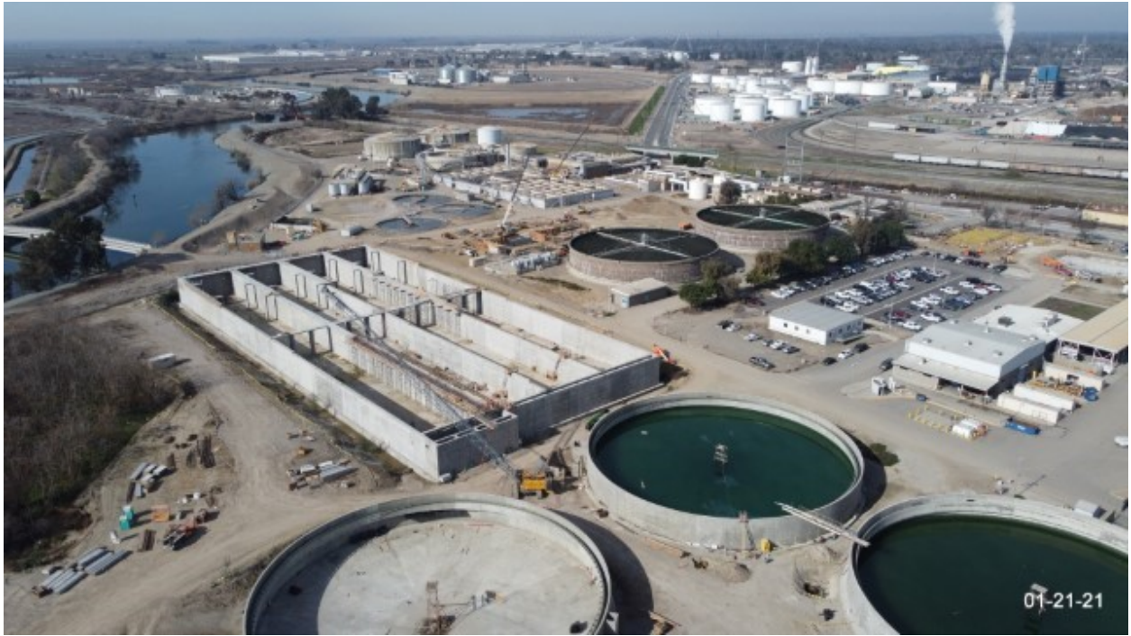
Aeration Basin looking west in January 2021.
