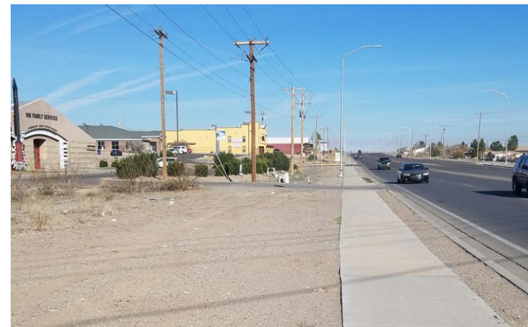
Figure 5-21 | Detached sidewalk along McNutt Rd
