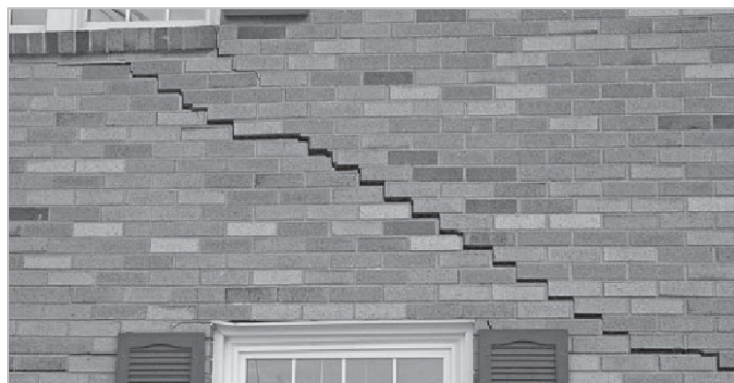
FIGURE 4-46 DAMAGE TO A HOME FROM MINE SUBSIDENCE
