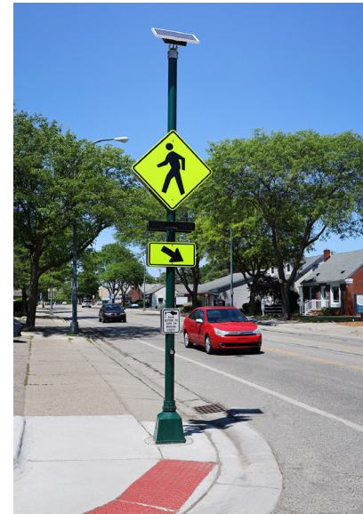
Figure 5-14. RRFB signal example
