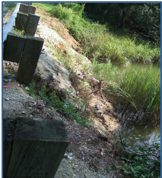
Figure H-9 Example of a poorly stabilized roadway construction project resulting in significant erosion directly into one of Murrells Inlet's tidal creeks. (Photo courtesy of Dr. Dan Hitchcock, Clemson University)
