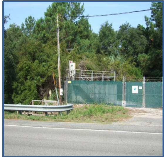
Figure G-1 Georgetown County WSD force main pump station equipped with the SCADA monitoring system. (Photo courtesy of Dr. Dan Hitchcock, Clemson University)
