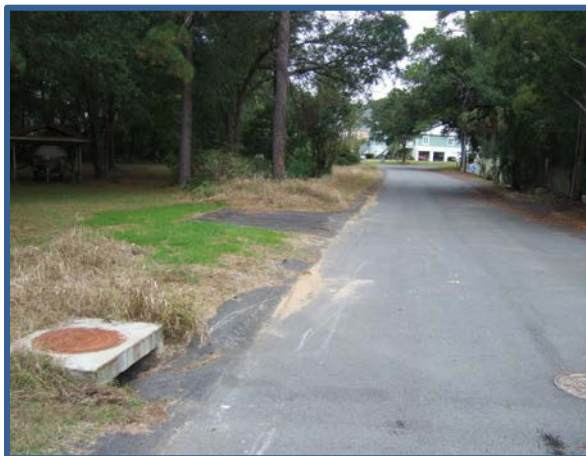
Figure C-9 Conventional storm drain which directs runoff untreated into the nearest waterbody (Photo courtesy of Dr. Dan Hitchcock, Clemson University)
