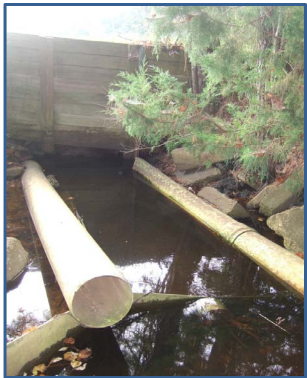
Figure H-1 A wide variety of stormwater management concepts have been tried in the past. This is the remnants of a chlorine contact chamber designed to treat water draining upstream of the Bike Bridge in Georgetown County. (Photo courtesy of Dr. Dan Hitchcock, Clemson University)
